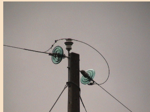
Box figure 2.1.1 SWER line, New Zealand
